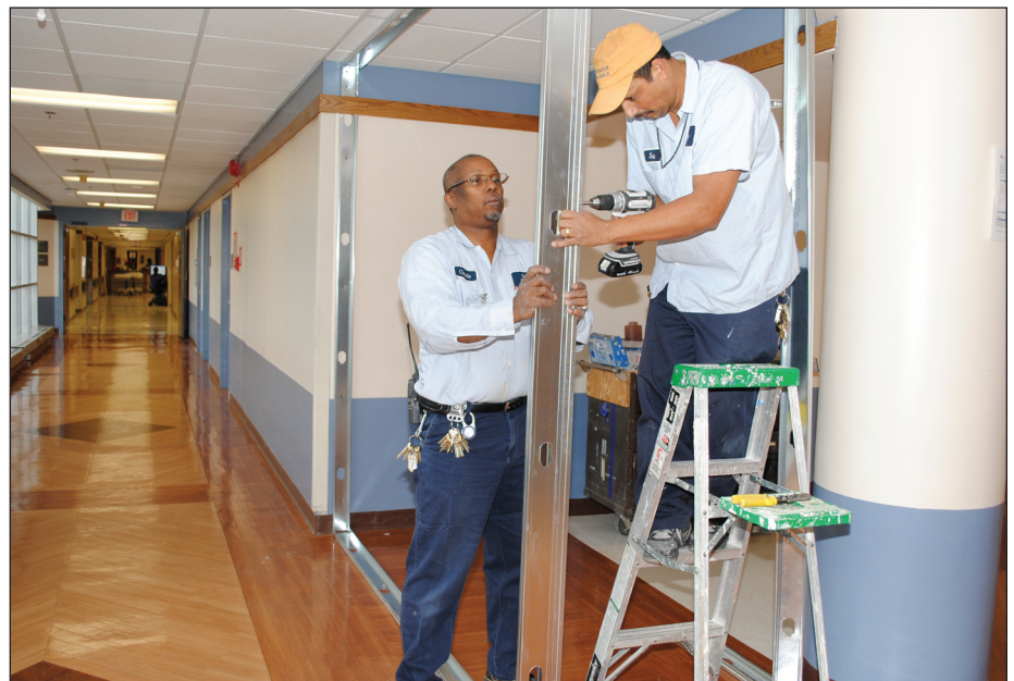
Construction Technicians Claude Williams and Jose Gonzalez , Engineering, build a new supply room on the fourth floor of the North Addition. This three-day project formerly would have been completed by a contractor, but having in-house staff do the work increases Hospital Center efficiency and reduces costs.
